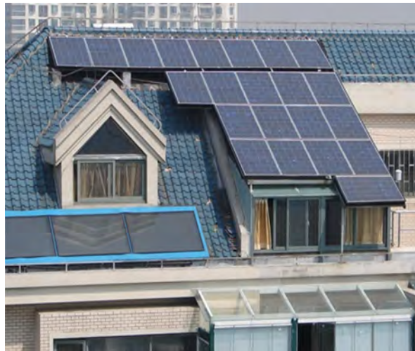
Figure 1-1 An example of a BAPV system [2]
